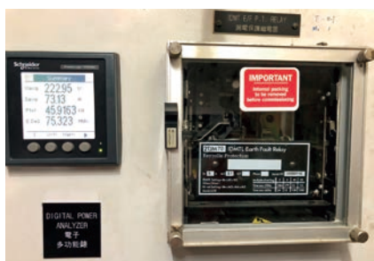
Power analyzer at Java Road 108 Commercial Centre
