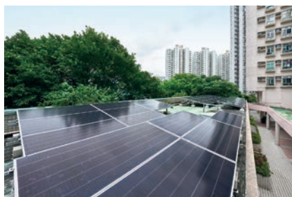
Solar panel at SSC
