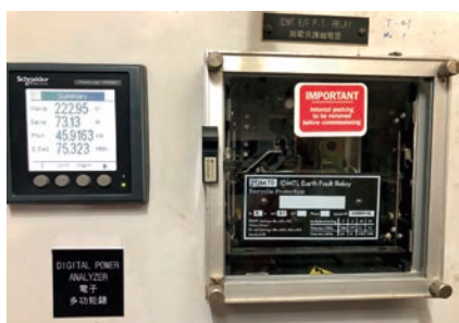
Power analyzer at Java Road 108 Commercial Centre
