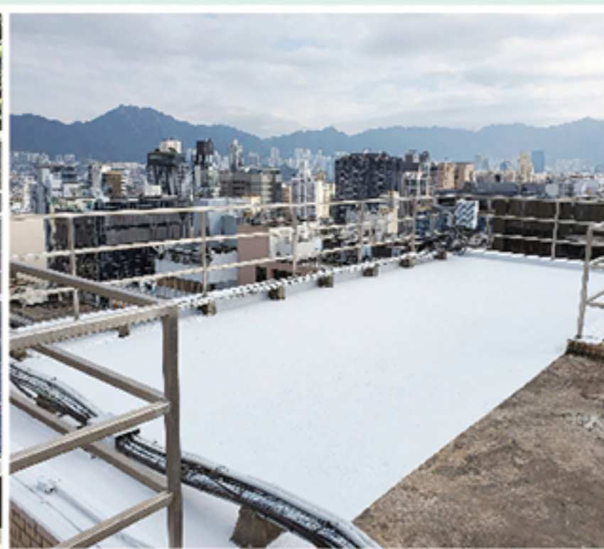
Application of coating on roof which help reflecting excessive solar heat from the roof surface and achieve energy savings
