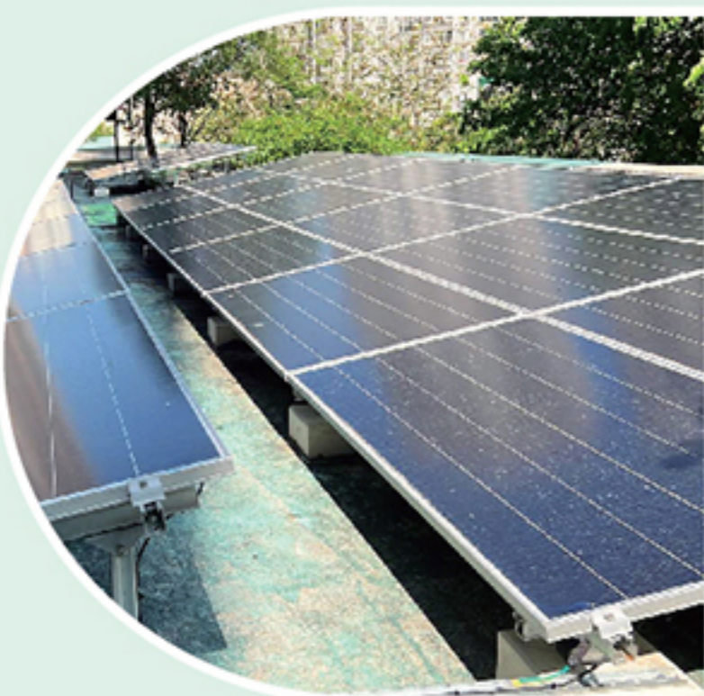
Sheung Shui Centre Shopping Arcade - Solar panel system
